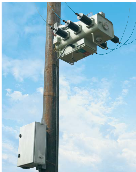
Automated Pole Mounted Load Break Switch
