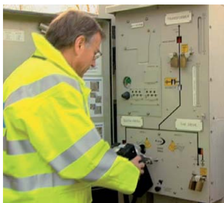
Automated Ground Mounted Ring Main Unit
