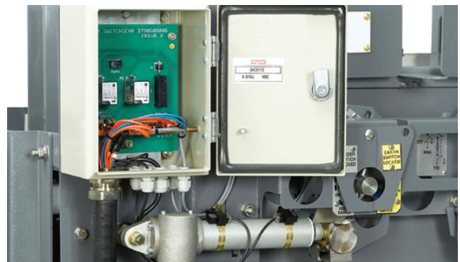
Automation actuator installed on ring switch
